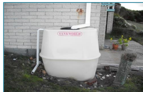
Figure 18 Large scale residential water butt. Source: Chris Digman
