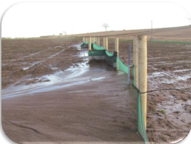
Filter fence. Note upslope spurs at plot edges to constrain lateral movement of sediment
