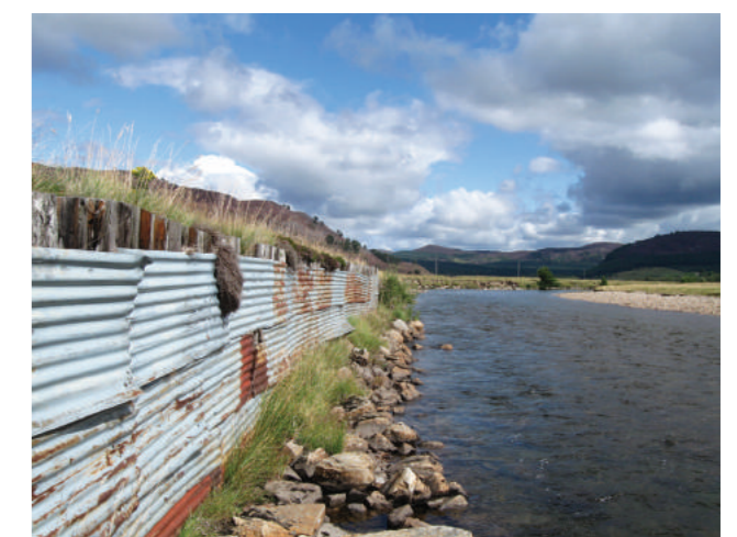
Figure 3.4 (Above) Bank reinforcement to stop natural erosion constructed from boulders on the Ewes Water, Dumfries and Galloway (© Martin Janes, RRC) and (Below) using corrugated iron and rubble on the River Dee, Aberdeenshire, Scotland. The River Dee bank reinforcement was removed in October 2015 to improve connectivity with the floodplain (© James Hutton Institute).
