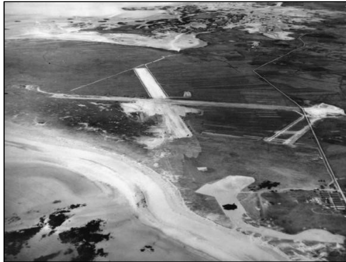
Figure 9.20: Oblique aerial view of RAF Benbecula, from west-south-west, while the runways were under construction in 1941-1942. The method used was known as 'sand carpet', which consisted of bitumen laid directly over compacted sand, resulting in a flexible surface. (© IWM (HU 92989))
