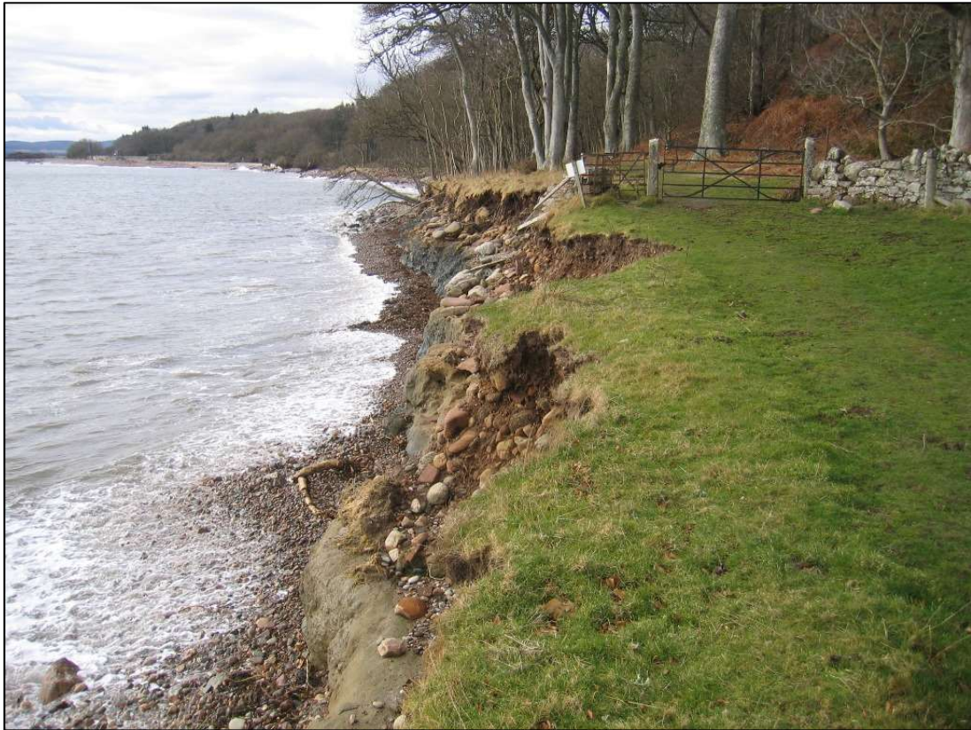
Figure 3.33: Evidence of erosion at Dunrobin Castle in 2000.
