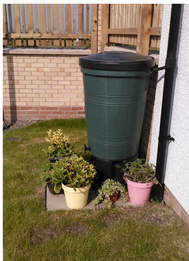
Figure B2.5. Rain barrel fitted at the show home. Image source: James Travers.
