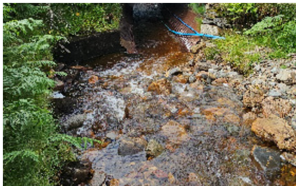
Photo 3F Culvert on the main channel upstream of impoundment. Looking downstream. Taken from river left.
