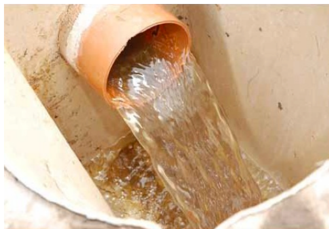
Figure 13 Clarified effluent from a septic tank.
